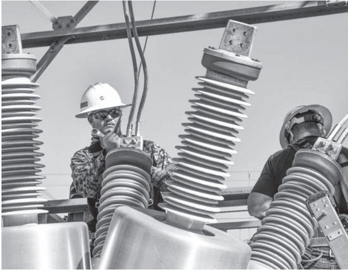
(Top) Brayden Johnson, apprentice electrician, tightens bolts on a 69-kilovolt breaker lead during a buss upgrade at Humboldt Switching Station Oct. 7.
