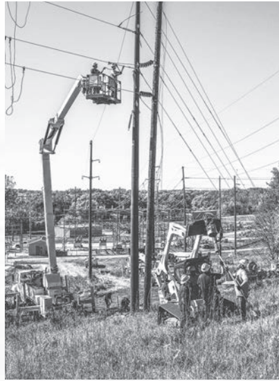
(Right) Corn Belt Power transmission crews secure anchors and guy wires on a new stack pole along the Humboldt to Webster line in October.
